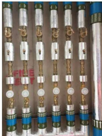
Figure 9. Internal metering set up for a multi occupancy building prior to IWNL meters being fitted
