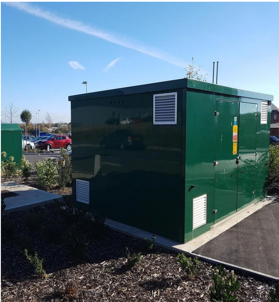
Figure 32. An example of how a large above ground installation should be finished
