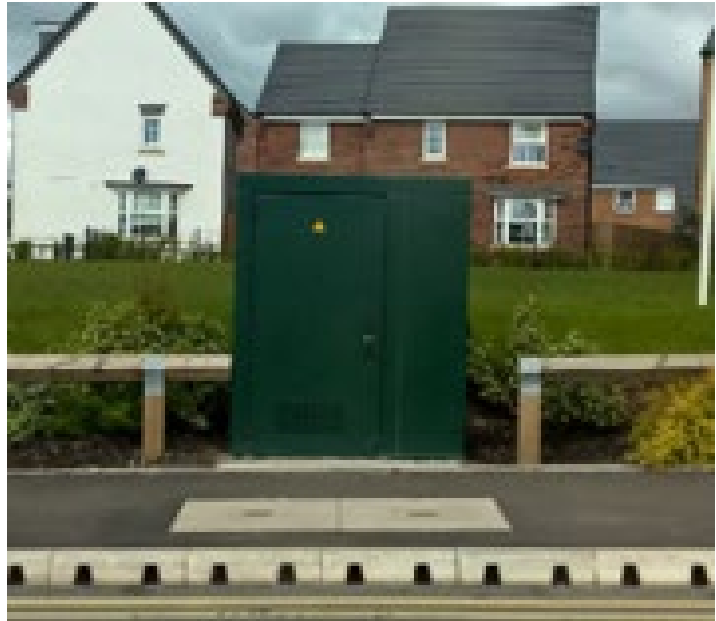
Figure 22. E.1 voice and data (non-FIRS) cabinet
