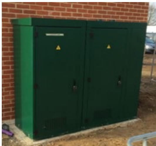
Figure 23. E.2 voice and data with FIRS cabinet
