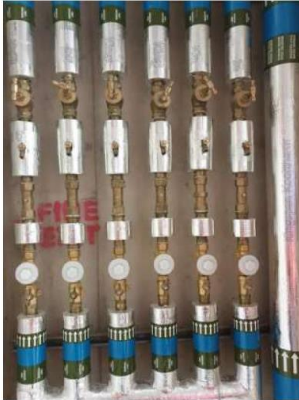
Figure 9 – Internal metering set up for a multi occupancy building prior to IWNL meter being fitted
