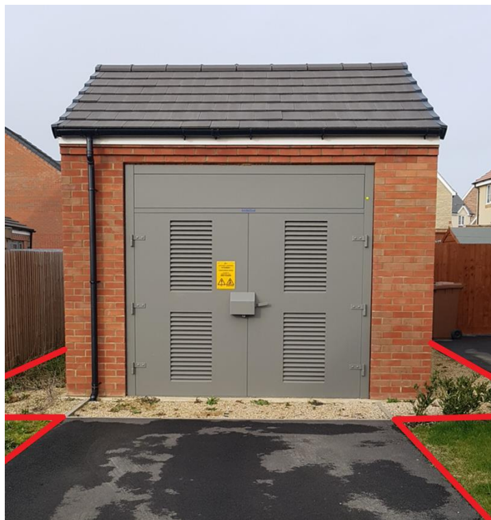
Figure 9 – A typical brick-built substation with at least 3m clearance to nearest property
