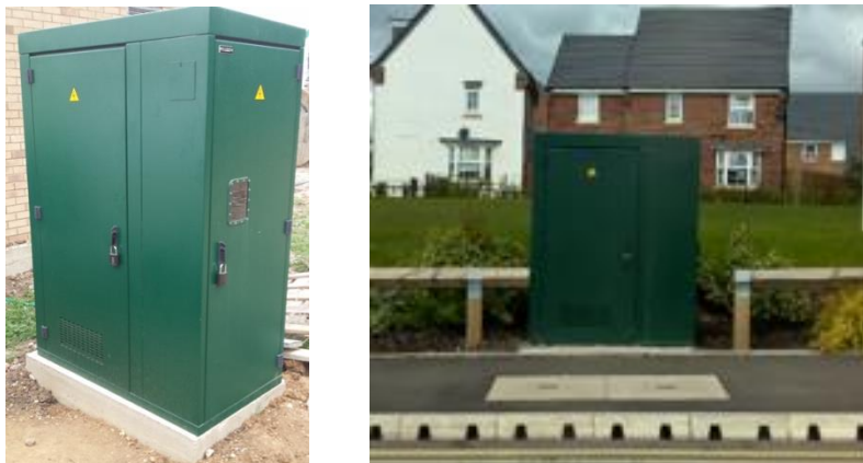
Figure 24 – E.1 voice and data (non-FIRS) cabinet
