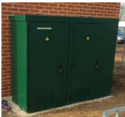
Figure 23 – E.2 voice and data with FIRS cabinet
