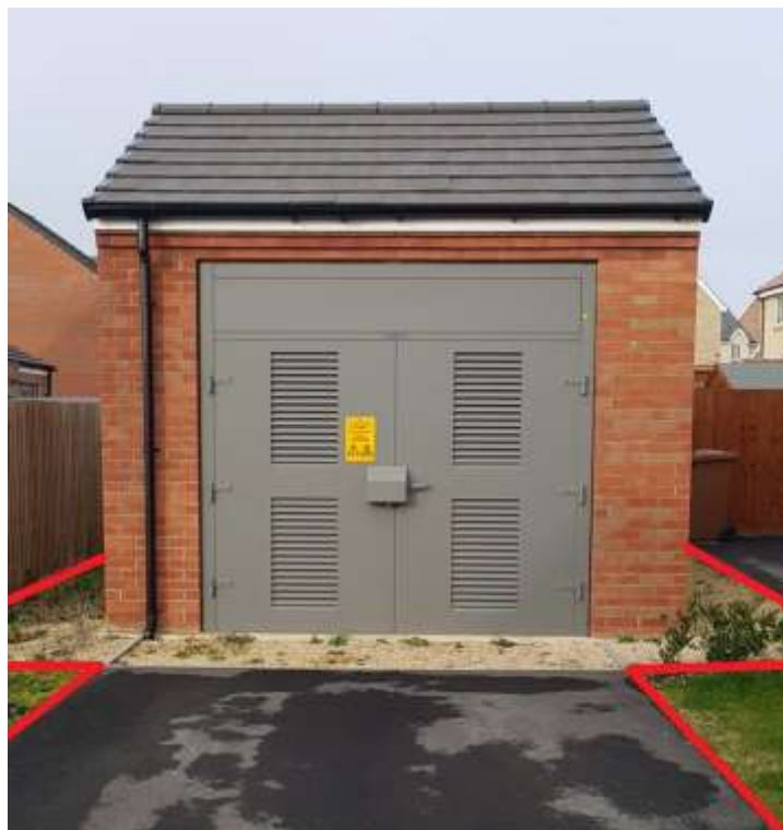
Figure 9 – A typical brick-built substation with at least 3m clearance to nearest property
