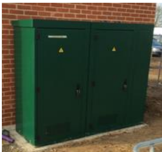
Figure 23 – E.2 voice and data with FIRS cabinet
