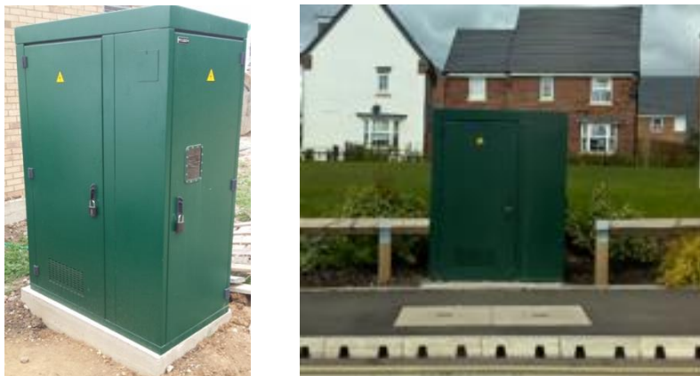
Figure 24 – E.1 voice and data (non-FIRS) cabinet
