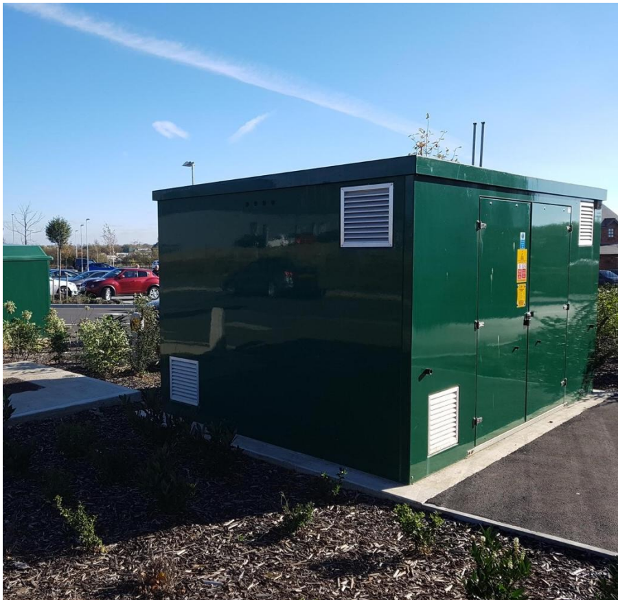
Figure 32 – An example of how a large above ground installation should be finished
